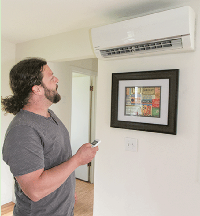
Dave Leterro uses the remote control to operate the ductless heat pump installed in the house he has been fixing up.
